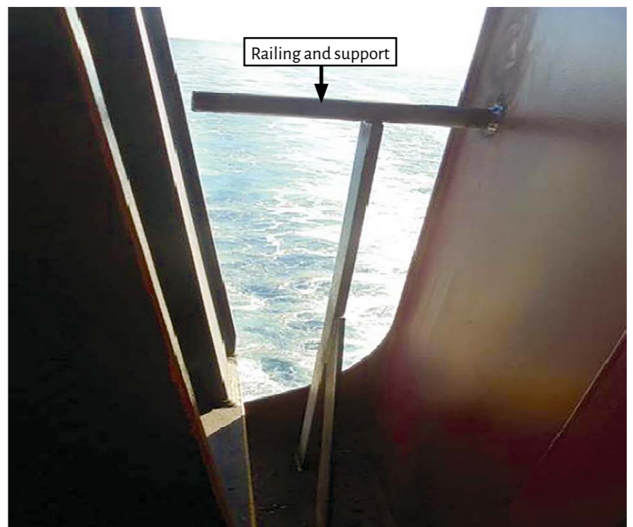
Figure 2: The guarded opening following remedial action
